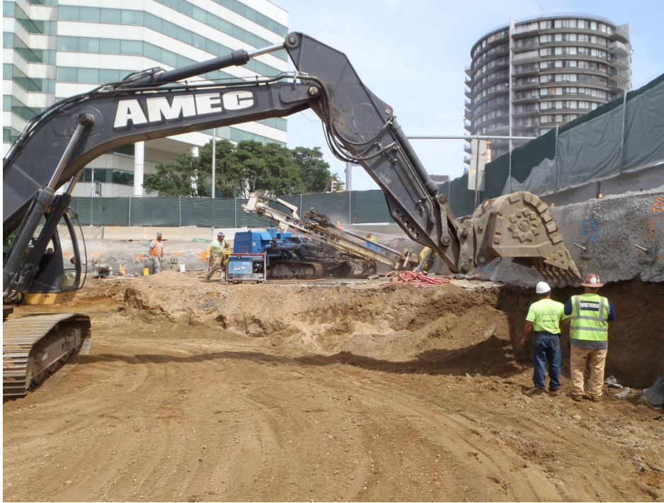
Figure 3.13: Photo. Excavation of soil lift during construction of soil nail wall. Photograph courtesy of Moretrench American Corporation.
