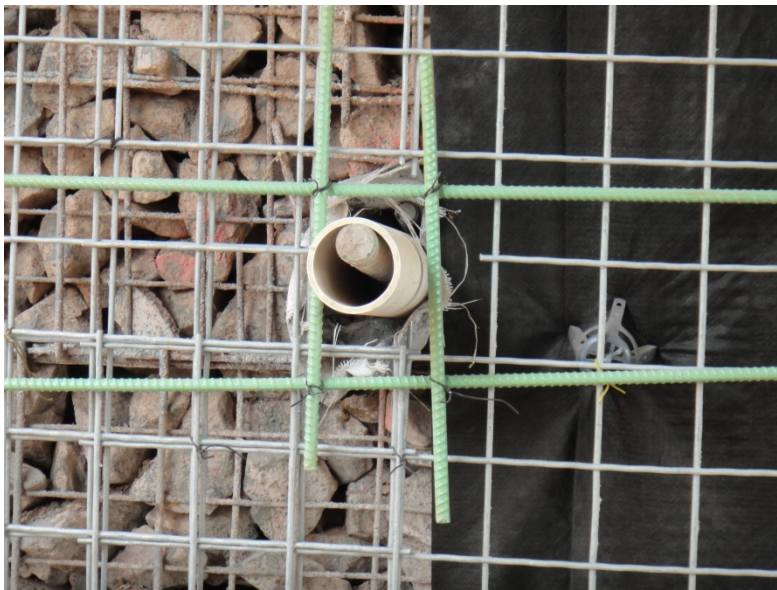
Figure 3.18: Photo. Shotcrete reinforcement including WWM and waler bars. Photograph courtesy of Ryan R. Berg & Associates, Inc.
